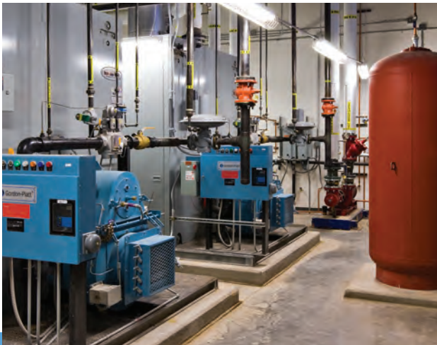
Bottom Left: High-efficiency hot water boilers
