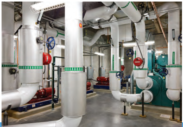
Bottom Right: High-efficiency chillers
